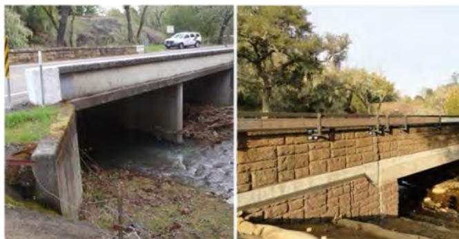
Capell Creek Critical Scour before and after
