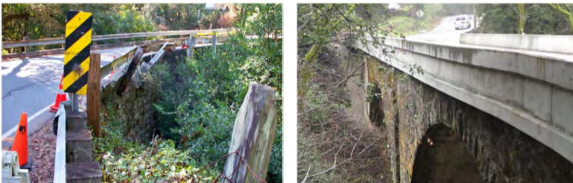
Figure 2. Saratoga Creek Bridge Rail before and after Repair
