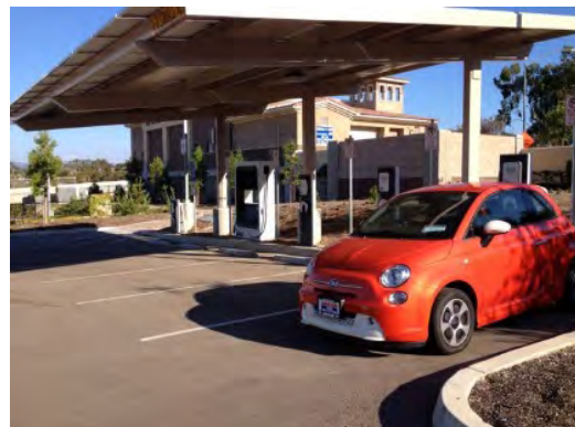
Figure 21. Public DC Fast Charging Station at the Del Lago Park and Ride in Escondido, CA
