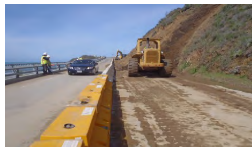
Unstable slopes and narrow shoulders along Route 101 to be cut to mitigate landslide risks.
