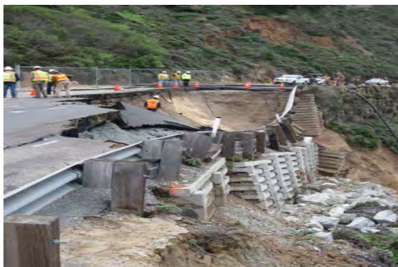
Figure 8. SR 1 in Monterey County before a slipout.
