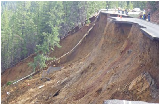
Figure 6. State Route 3 in Trinity County before emergency opening repair of a major slipout following intense rainfall in March 2016.
