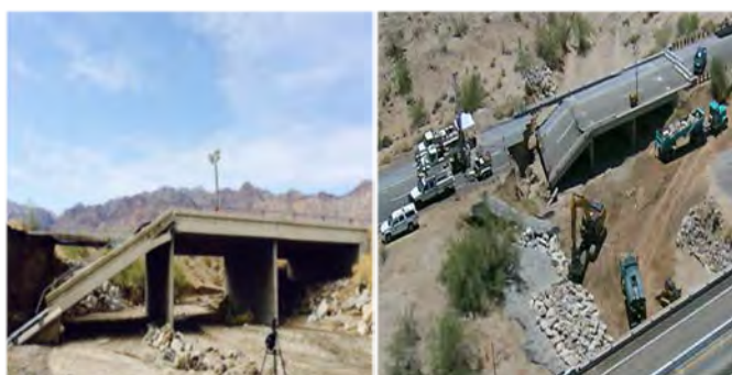
Interstate 10 Tex Wash Bridge Damage before Replacement
