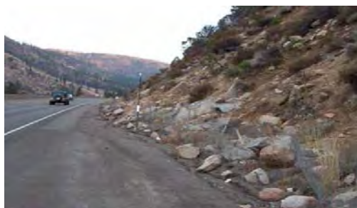
Figure 12. Catchment Ditch site along Interstate 80 to mitigate future rock slides.
