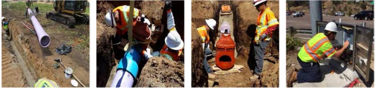
Figure 20. Recycled water project designed to improve water conservation using SMART controllers that enable efficient water usage to maintain roadside landscaping.
