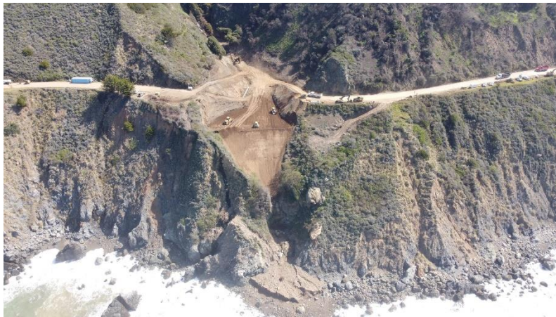
Figure 5-3. SHS Big Sur, Highway 1 Rat Creek landslide (Source: Caltrans)
