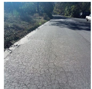
“Failed,” Marshall Lane
