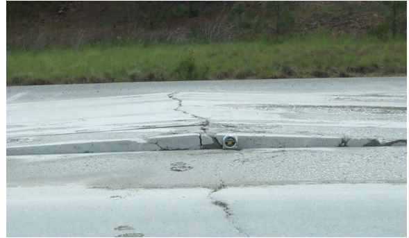
Figure E3. Example of concrete blowup.
