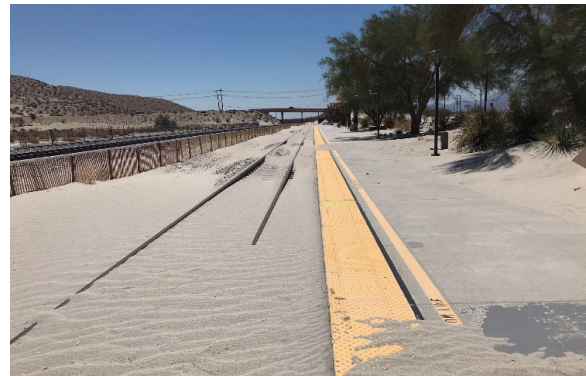
Existing condition: Blowsand at Amtrak's Palm Springs Station
