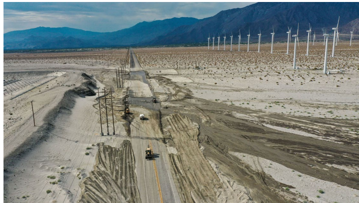
Crews clear mud and sand off Indian Canyon Drive in Palm Springs, CA – September 12, 2022
