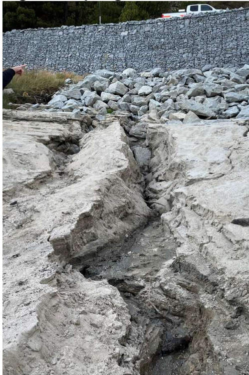
Figure 2: Spring and its Washout
