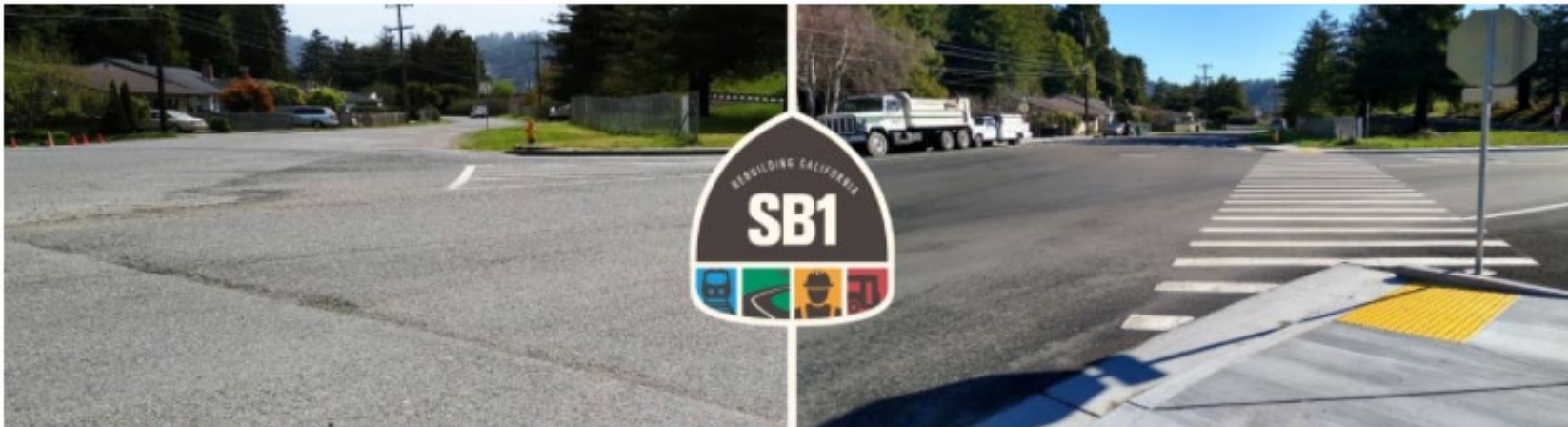
In the City of Rio Dell, Caltrans District 1 installed new curb ramps, sidewalks, crosswalks, and bike lanes to improve safety.
