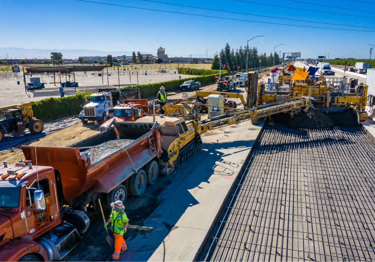
Route 99 concrete pavement- Fresno County from the City of Selma to Kingsburg
