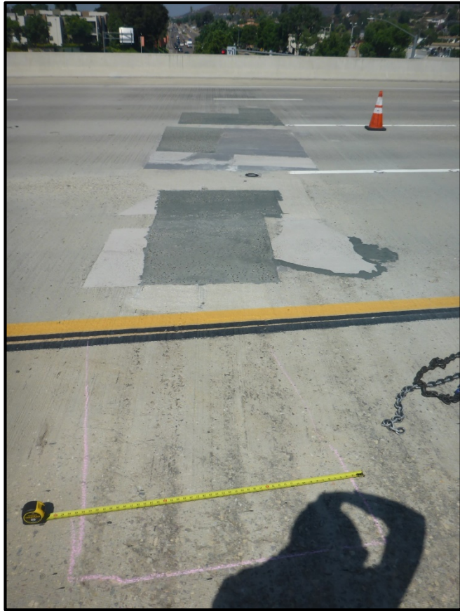
Before - POOR Condition Deck
