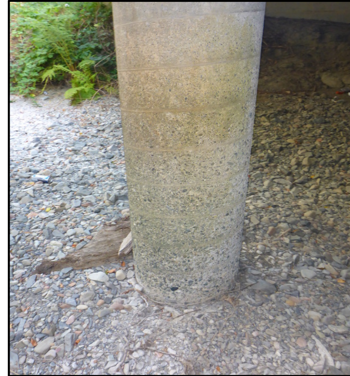
Bridge column with cosmetic abrasion
