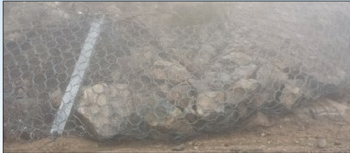
SR-18, January 2017. Debris stopped by rock barrier
