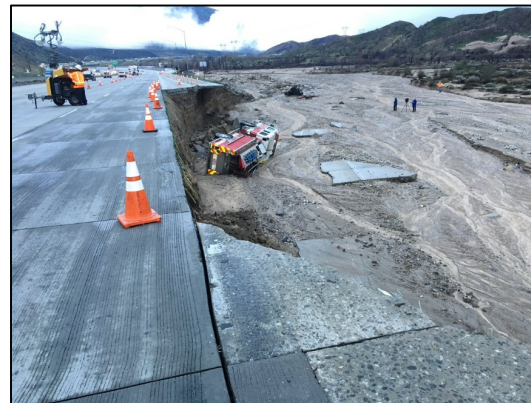
I-15 Washout, February 2017 District 8
