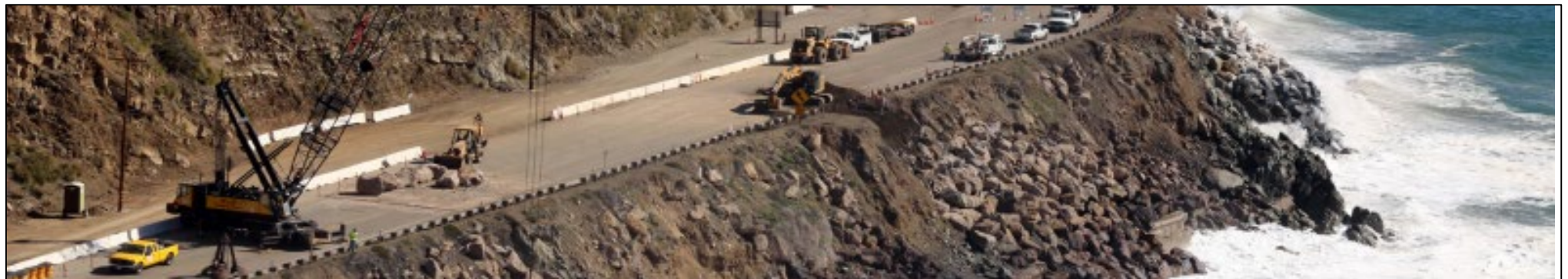
Pacific Coast Highway slide damage
