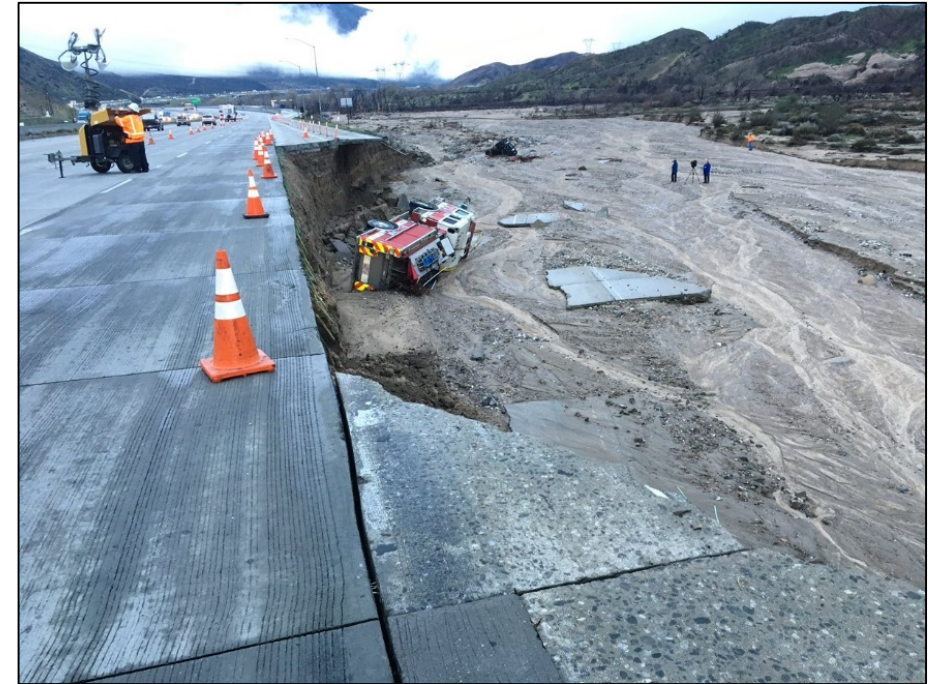
I-15 Washout, February 2017 District 8
