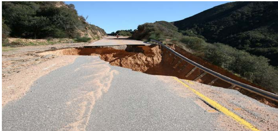
Major erosion event along 101 in need of repair
